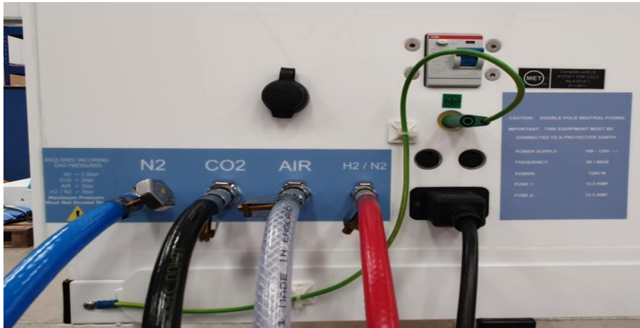
Figure 3: Gas and electrical connections
