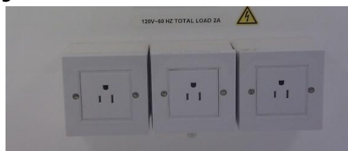
Figure 116: US Internal Power Sockets
