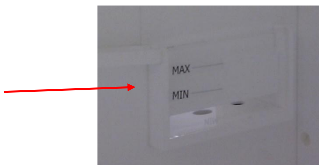
Figure 256: Water tank internal level indicators
