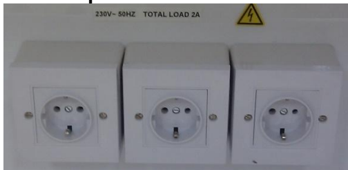
Figure 14: European Internal Power sockets
