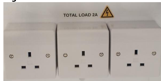
Figure 15: UK Internal Power Sockets
